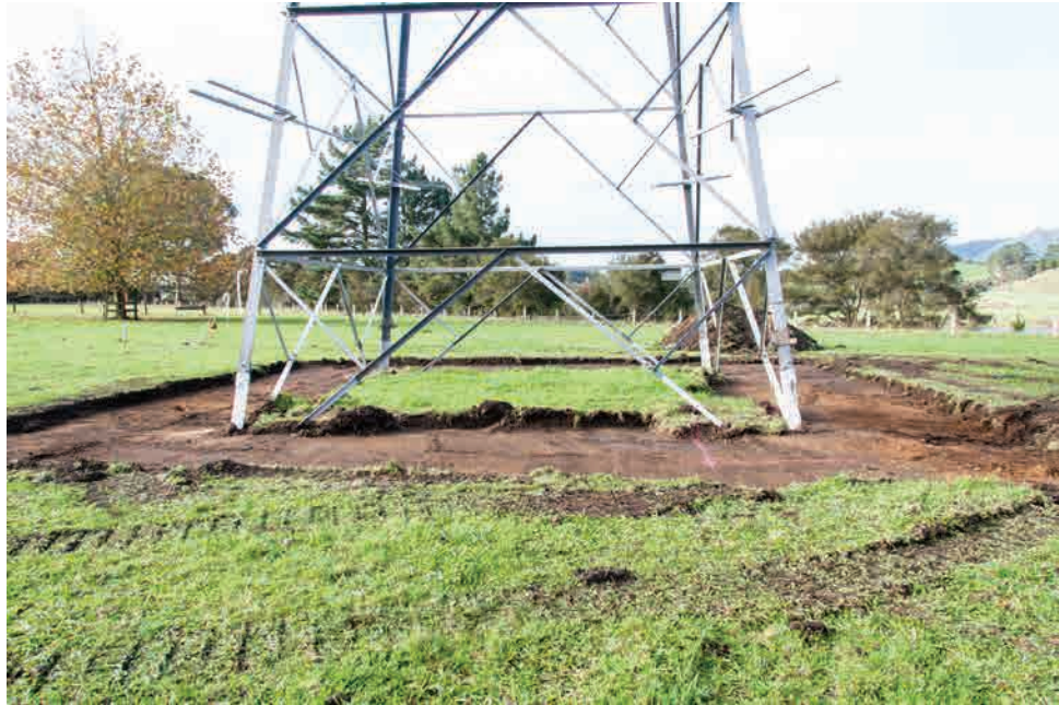
3. Tower A 0051 showing the format of excavation with a single trench surrounding the tower and footing cuts about to commence, facing south east.
